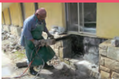
James Sutton of Dixie Concrete Cutting Co. cuts out the stone from a window on Area B.
