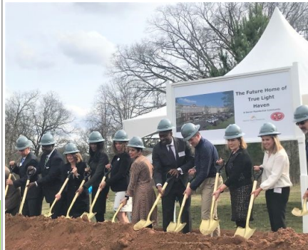
Dignitaries turn the first shovel full of dirt for the new True Light Haven apartments.
